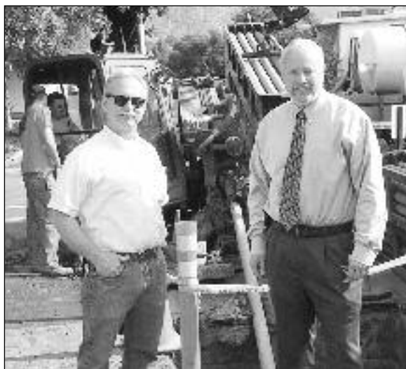
Senior Project Manager Larry Grubbs and Engineer George MacMullin are overseeing the $9.9 million project to modernize UCR's infrastructure.
